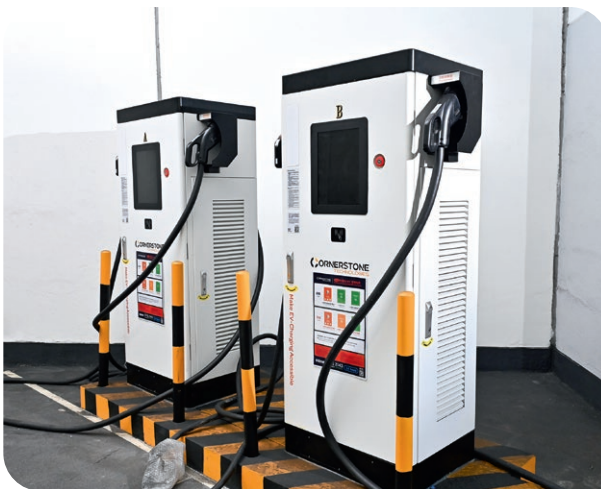
警察總部大樓內的電動車充電站。 Charging points for electric vehicles at the Police Headquarters Complex.
