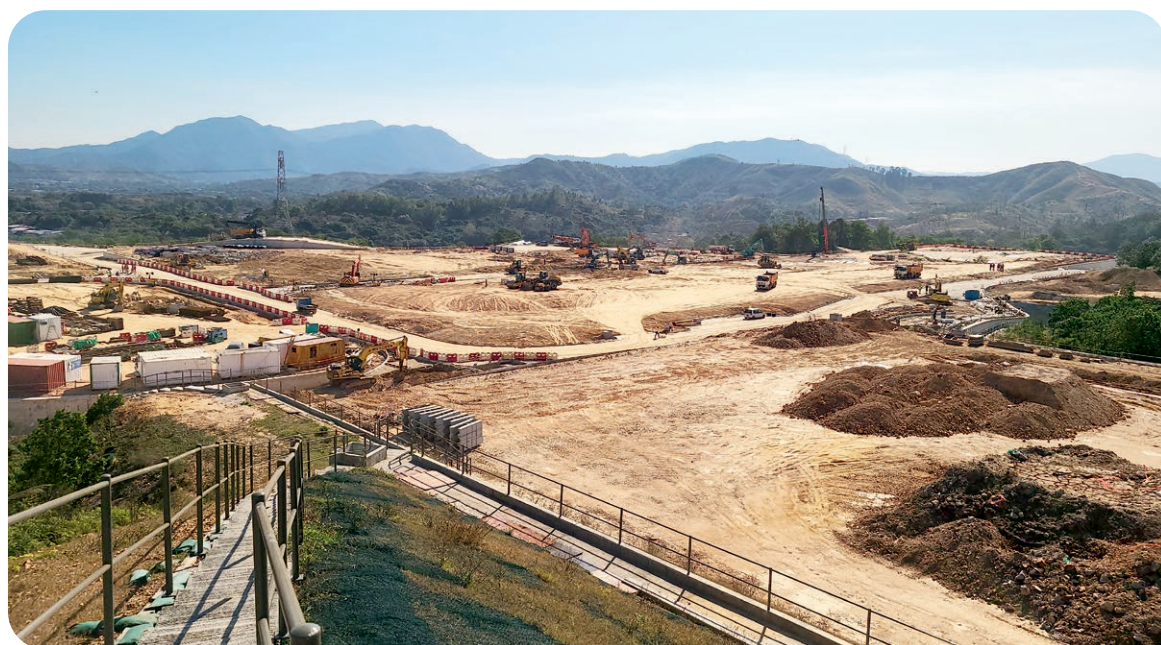
缸瓦甫警察訓練設施的建造工程於十二月展開。 Construction of the Kong Nga Po Police Training Facilities began in December.
